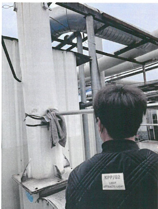
污水处理废气排气筒出口(FQPK-0006)G6
