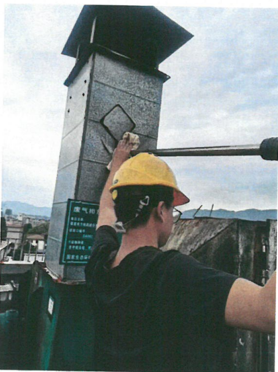
污水处理废气排气筒出口(FQPK-0005)G5
